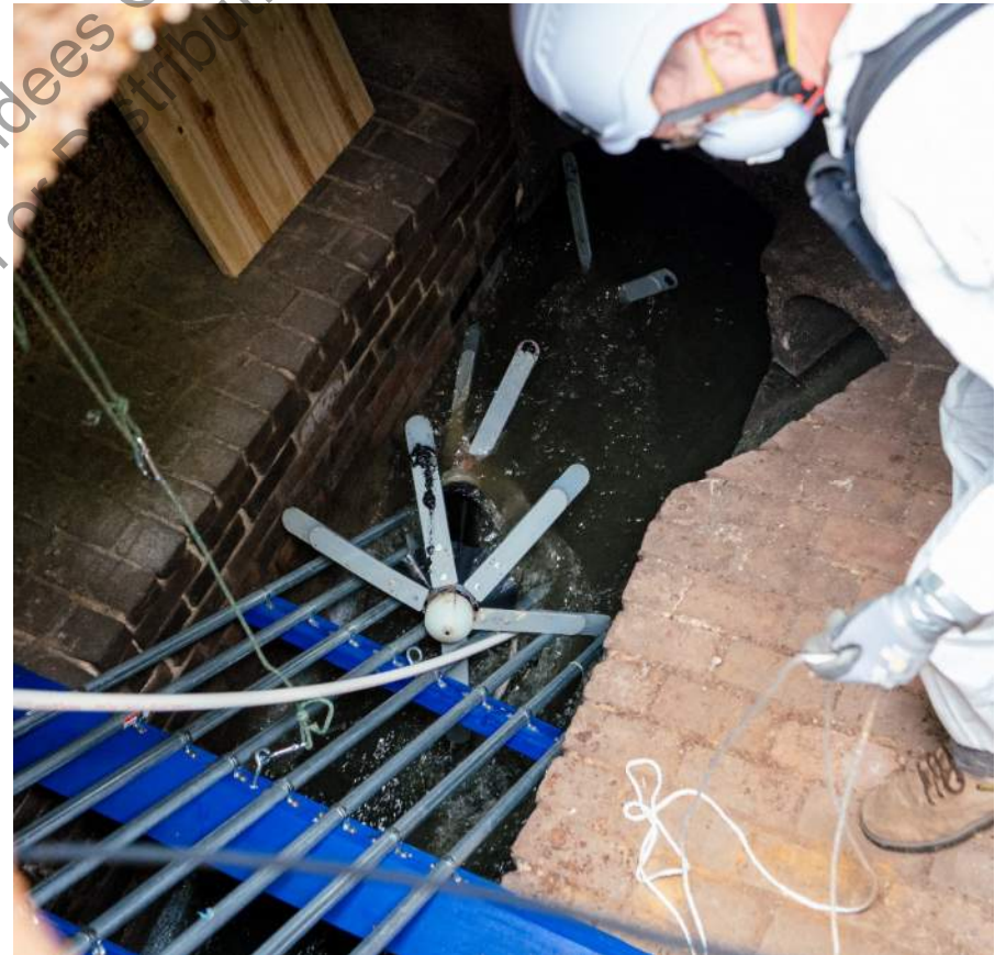
Inspection device arrives at extraction
