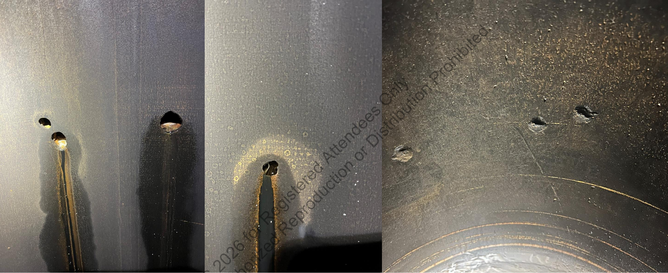
Approximately 5 Through Walls Total
