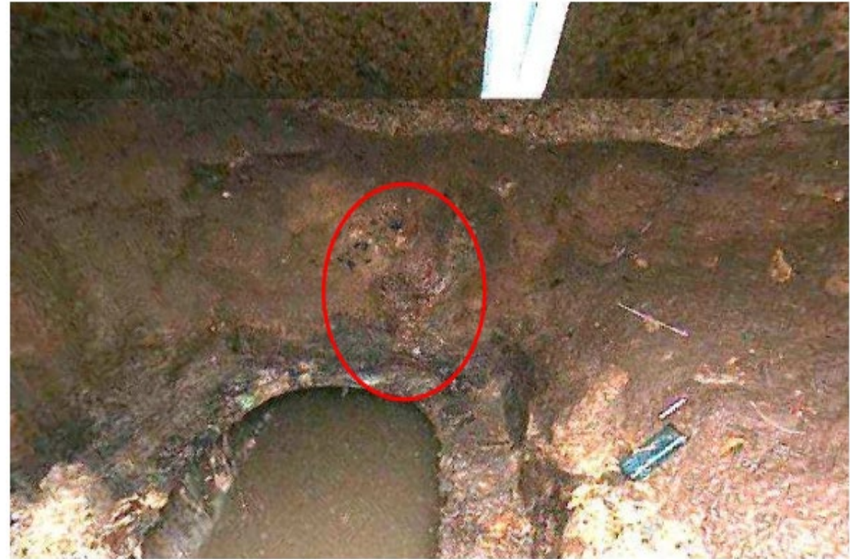
Infiltration Weeper – MACP Score 2
