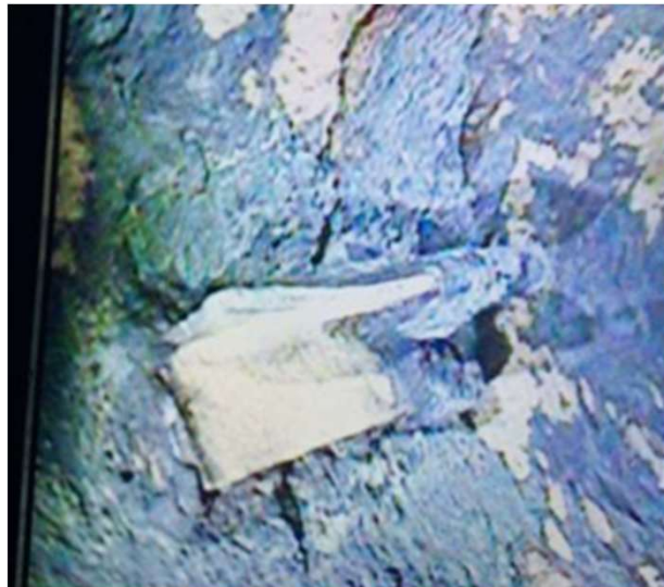
Protruding Angle Iron
