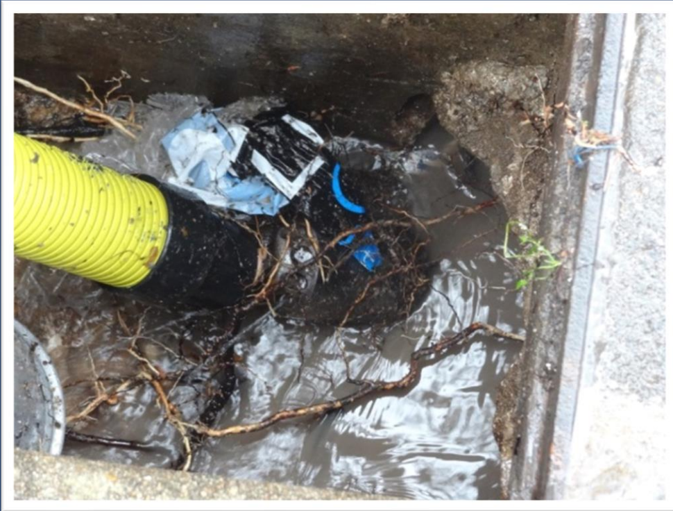
Root intrusion in shallow lines.
