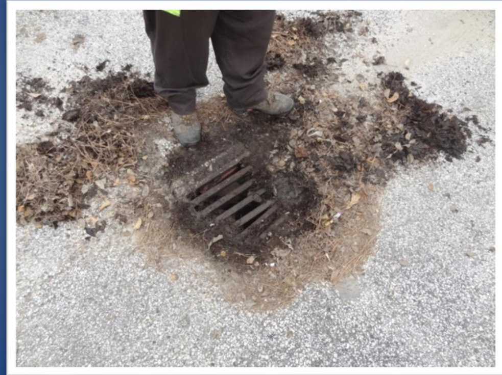
Accumulation of debris in and on catch basins.
