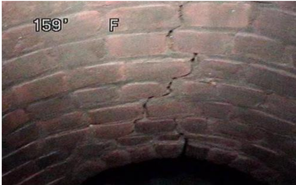
Wall Interior (WI) - Fracture Longitudinal (FL)
