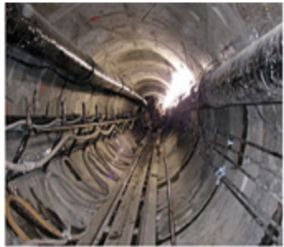
Tunneling for installation of the new East Central Interceptor Sewer. Photo courtesy of the City of Los Angeles
