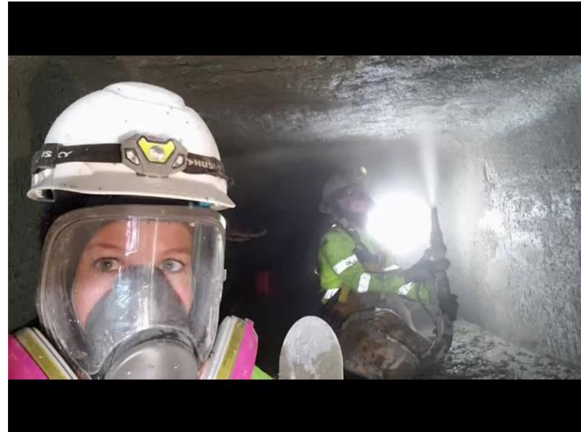
Michelle Beason working alongside the crew, 9' x 6' Box Sewer Rehab Project, San Francisco, CA, 2018.
