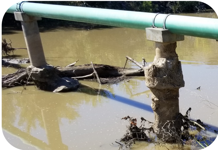
Aerial crossings risk debris hitting piers
