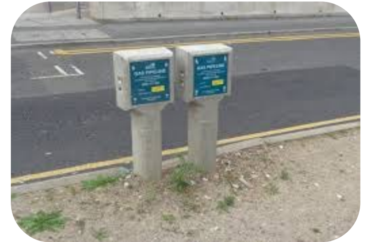
Cathodic protection (utility dependent)
