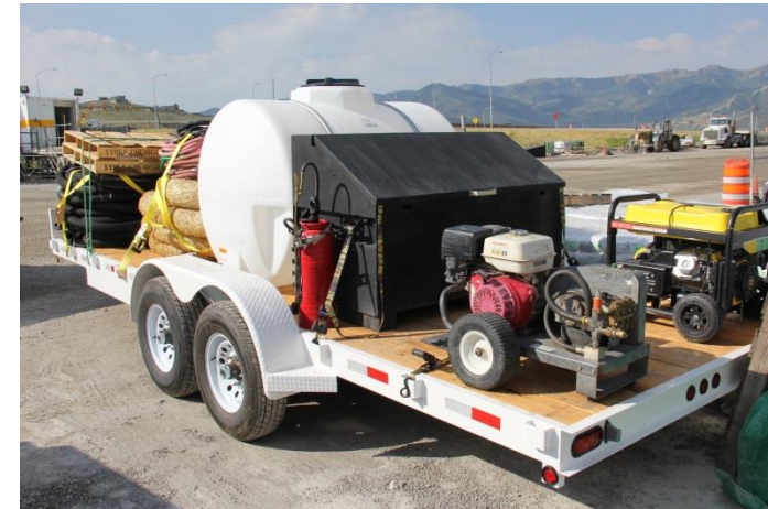
Support Equipment (375 CFM Compressor not Shown)
