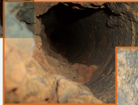
Partial tuberculation removal
