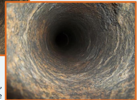
Full tuberculation removal, bitumen liner visible
