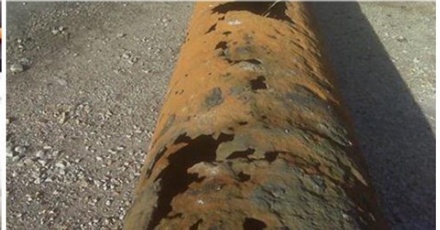
1975 Ductile Iron Pipe Southern New Hampshire
