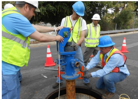
This custom hydrant guides the rope past a seal. By using clamps to hold the hydrant in place, flange patterns don't have to match.
