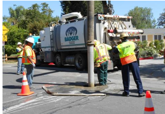
Vacuum excavator was performed using a high-volume unit equipped and water jet lances.
