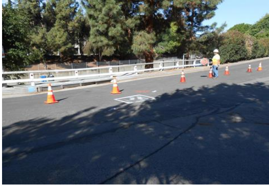
Traffic control by LADWP. The hole location was pre-marked and cleared for excavation. The location is the intersection of Valleyheart Drive and Ethel Avenue.
