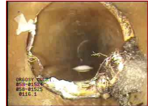
Sewer Pipe in Baton Rouge area BEFORE CCTV Cleaning
